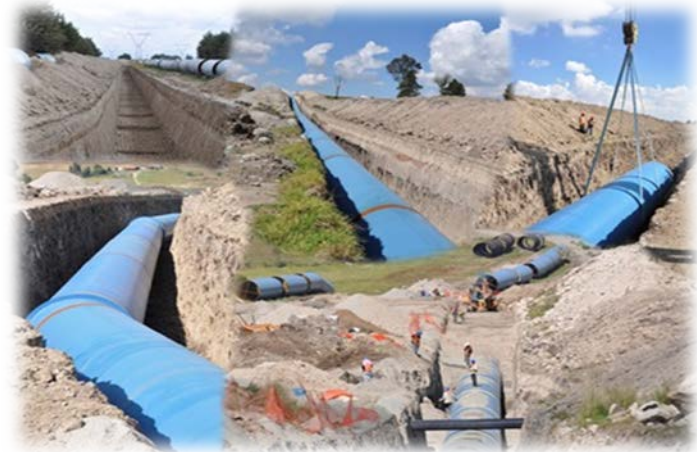
Water network (Cutzamala - México)
