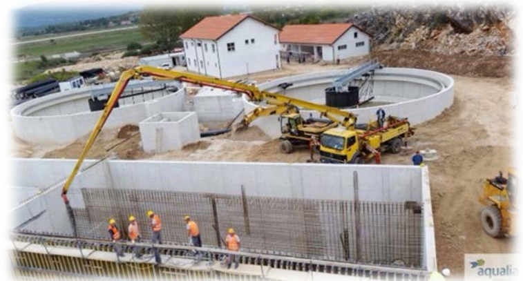
Waste water tratment plant (Montenegro)
