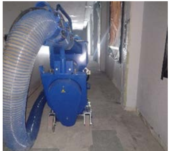
Negative pressure and air removal (dynamic confinement/depression). Fume test
