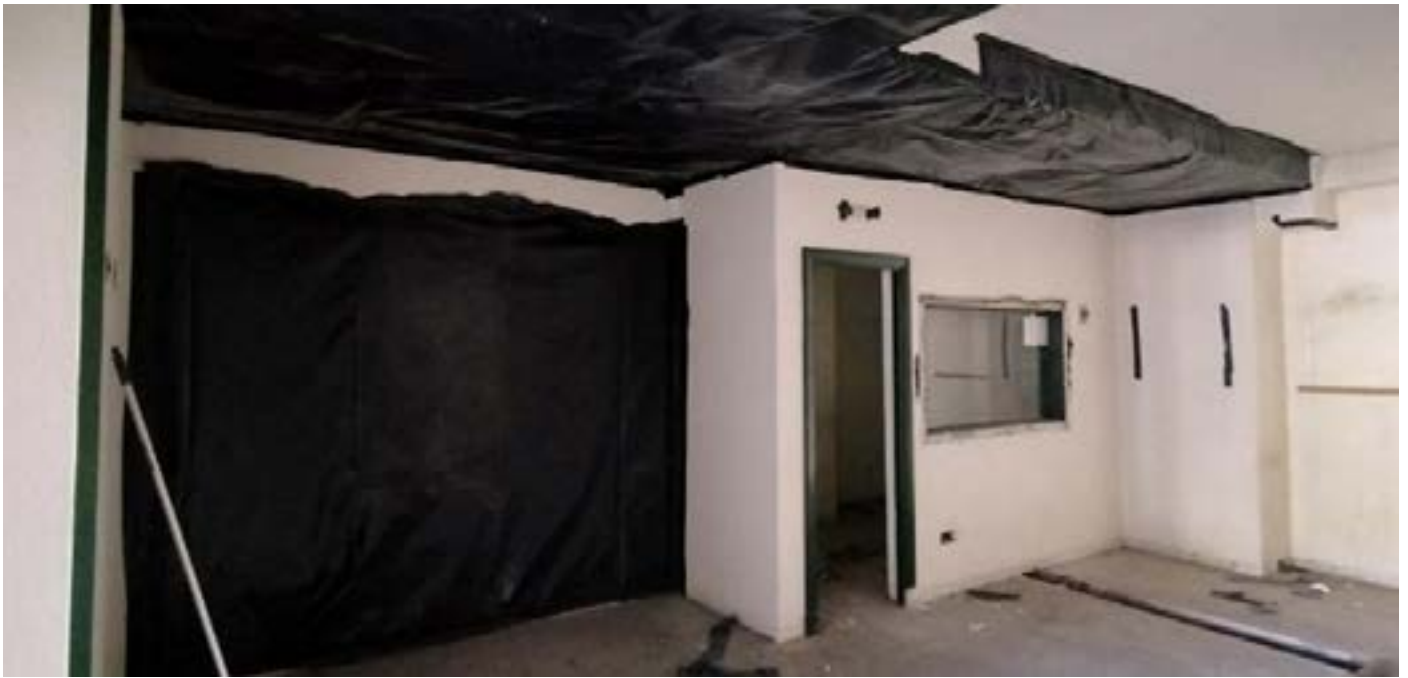
Removal of all materials that may hinder work and are likely to be contaminated. Execution of barr and formation of barriers and confinement
